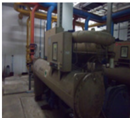
Screw Compressor Chiller
